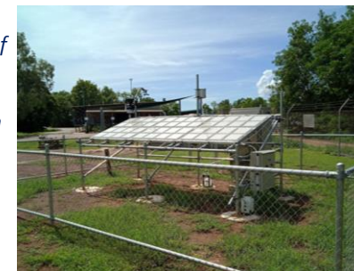
Artificial photosynthesis panels installed in Darwin, Australia
