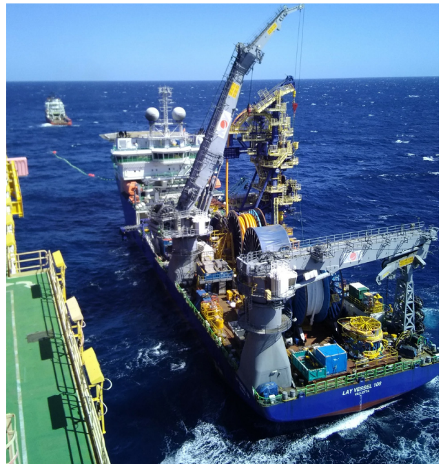
McDermott's LV108 supported post-lay activities, including the installation of new risers during the maintenance turnaround campaign.
