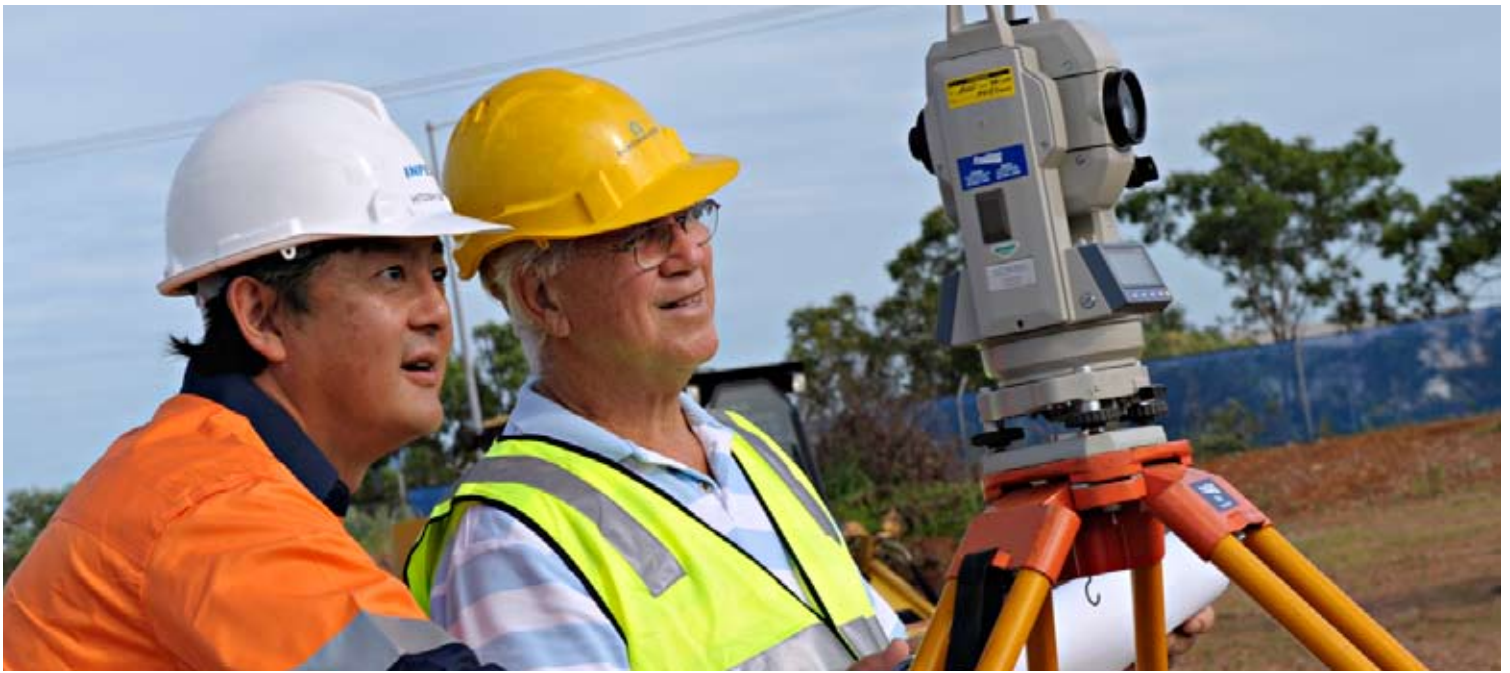
INPEX Director of Corporate Coordination Hitoshi Okawa and Larrakia Development Corporation Chairman Koolpinya Barnes inspect the Larrakia Trade Training Centre site.
